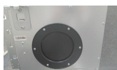
Outside air inlet reservation
